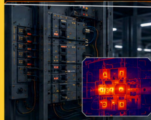
POWER PANEL MONITORING 配電盤監測
